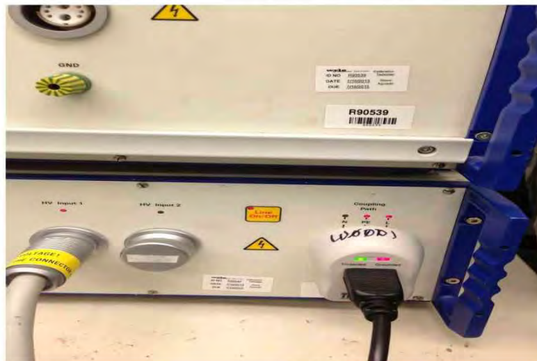
Photograph 12: ES&S FL EVS 4.5.0.0 Lightning Surge
