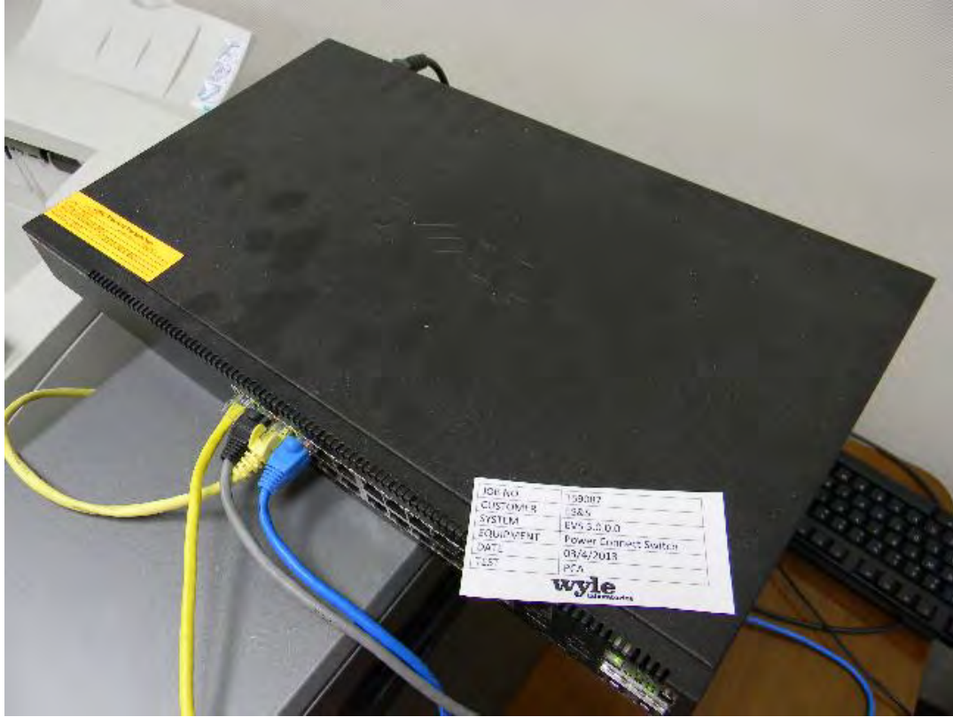
Dell Power Connect Switch
