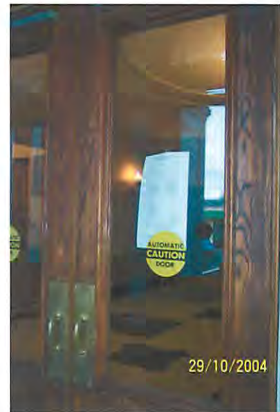
FIGURE 23 AN “ACCESSIBLE” DOOR THAT AUTOMATICALLY SMACKS INTO A VOTER WHEN APPROACHING THE POSTED VOTING INFORMATION
