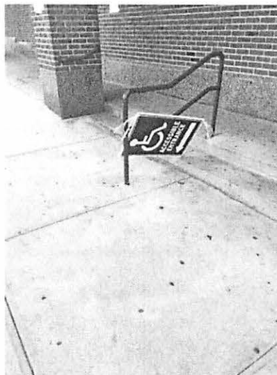
Photo #16. PS 173 – Poorly attached sign for accessible entrance, now useless for directions.
